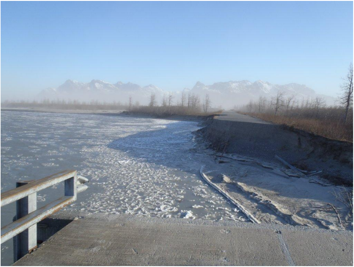
Figure 1 – October 26, 2012 road breach (approx 185') looking east
