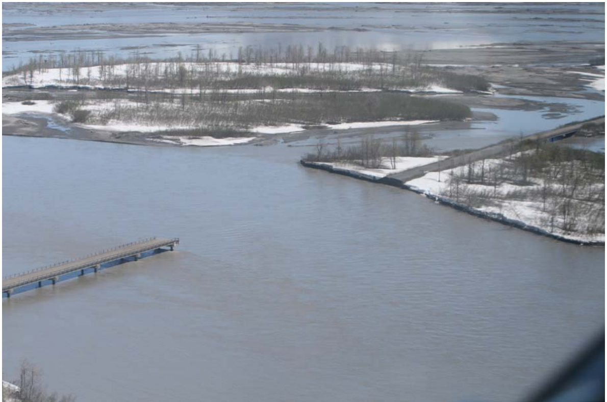
Figure 2 – June 9, 2013 road breach (approx 800') east side of Bridge 339
