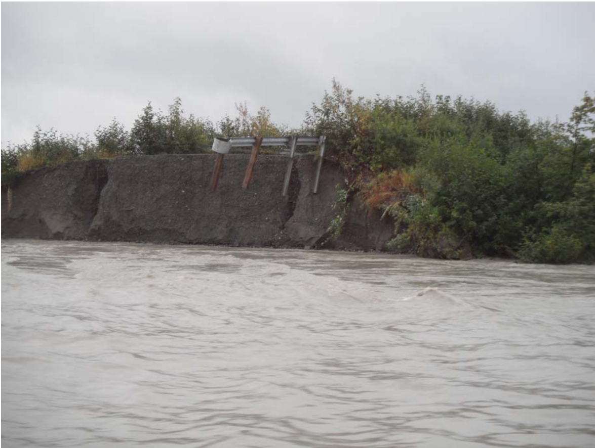
Figure 5 – September 10, 2013 road breach (approx. 1055') looking northeast at Bridge 340's approach guardrail
