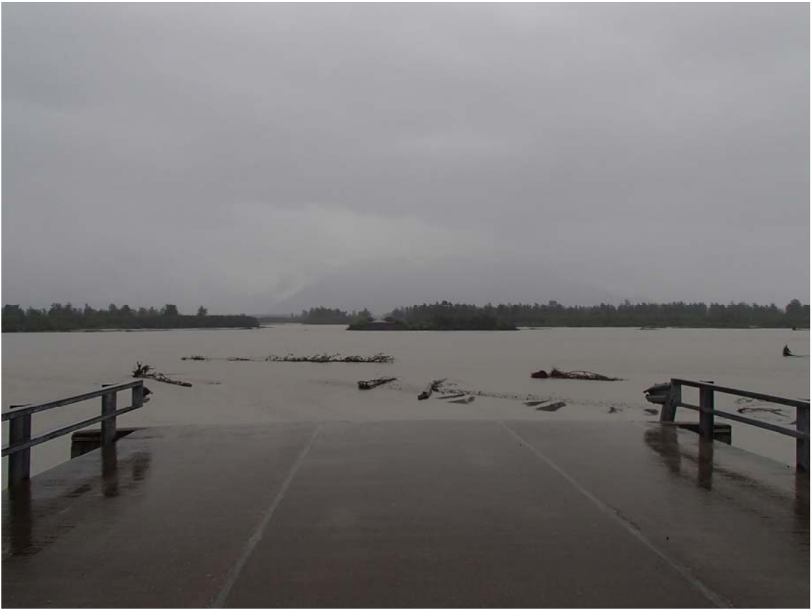
Figure 3 – August 21, 2013 road breach (approx 972') looking east
